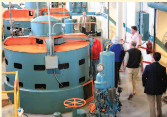
Canal Authority members tour Sibley hydroelectric plant.
